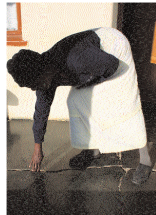
A woman from a community forum points to the cracks in her houses caused by the mining operations in the vicinity.
