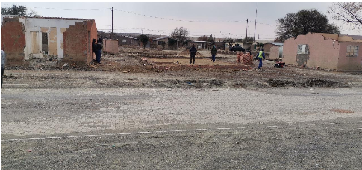
Figure 8 A new house being built close to the ones that were damaged by the sludge
