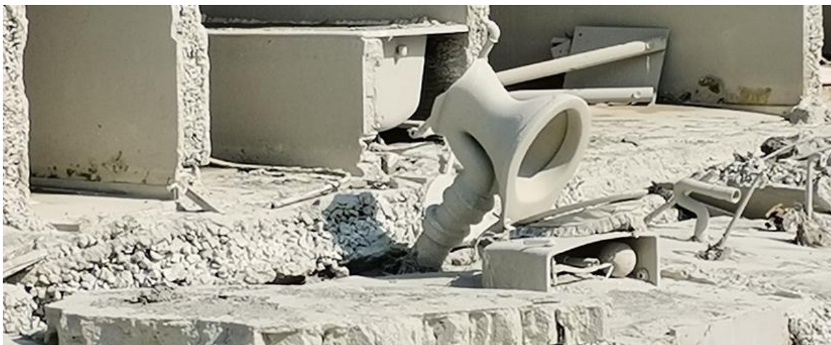
Figure 11 Sewage infrastructure in some private homes and in the municipality was swept away (Photo Brown Motsau and David van Wyk)
