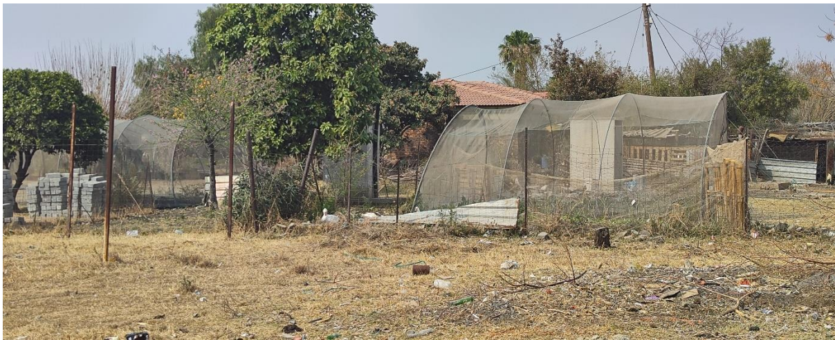
Figure 46: Vegetable tunnel frames in reality - most are in various states of dereliction
