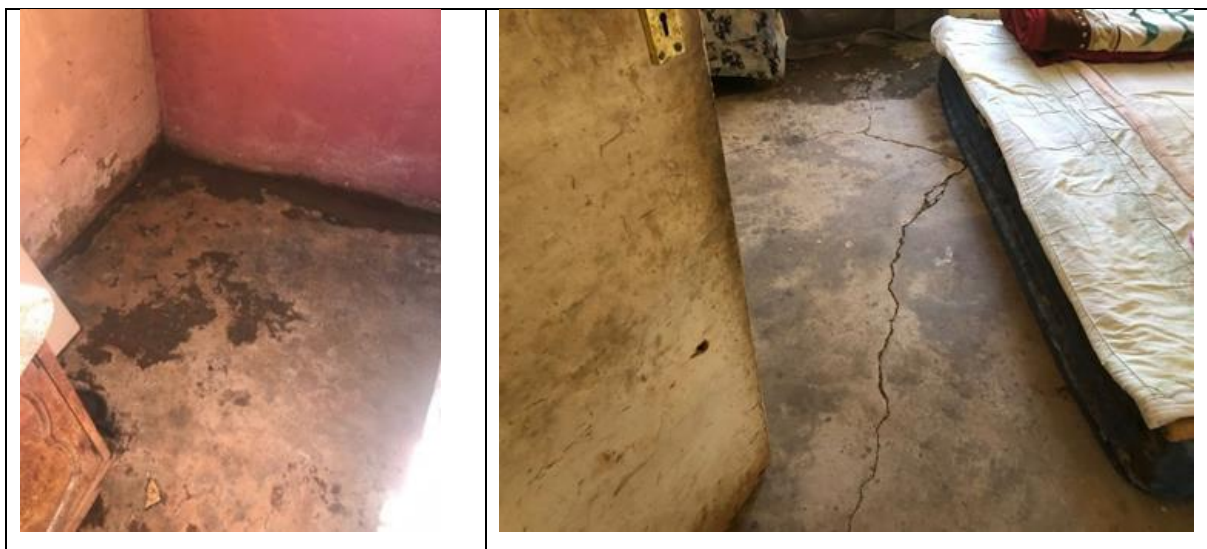
Figure 34: Photos showing cracked housing and damp in houses in Wonderkop (Photo: community member)
