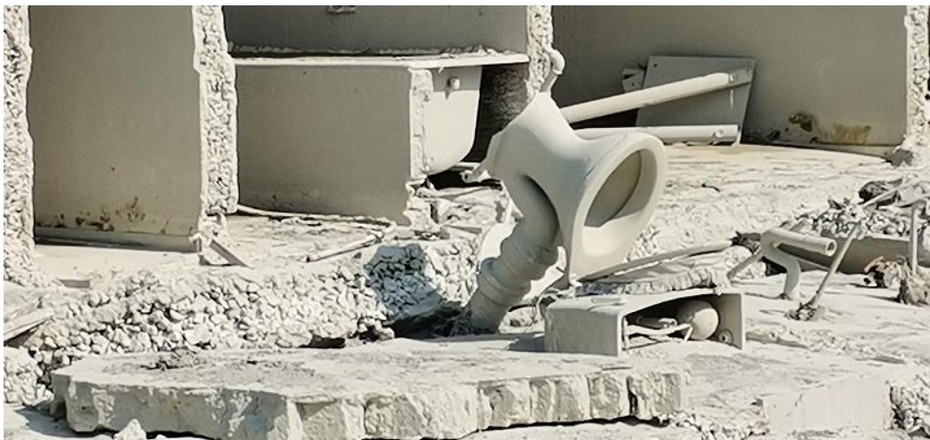
Photo 7 Sewage infrastructure in some private homes and in the municipal infrastructure was swept away (Photo credit Brown Motsau and David van Wyk)
