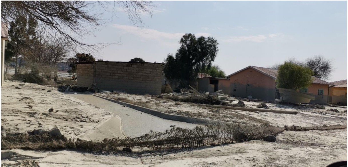
Photo 4 Only thing left of the houses in the front of the photo are their foundations, Charlesville (Photo credit Brown Motsau and David van Wyk)
